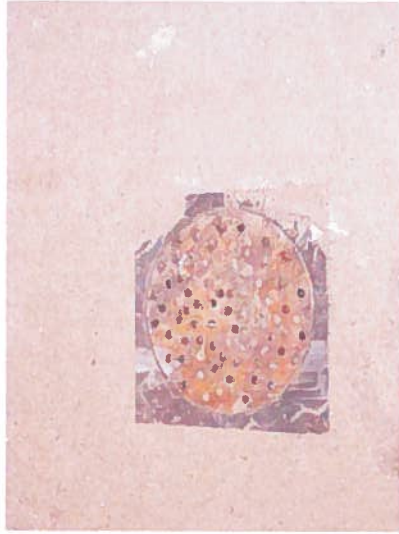
FIGURE 17: Several small diameter area drains are observed within the alley. These appear to be in poorly maintained condition with limited capacity.
