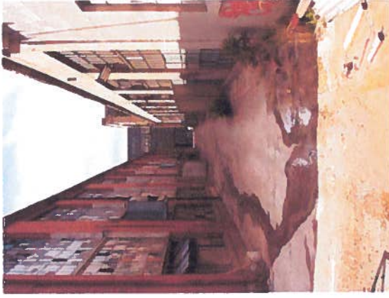
FIGURE 14: A narrow alley lies between the Blacksmith Shop and a CMU Warehouse to the west. This area lacks positive surface drainage. Surface drainage appears to discharge to an antiquated storm drain system and/or French drains. In either case, the existing facilities appear to be unmaintained and in disrepair. Replacement with a private storm drain connecting to Second Street SW is recommended.
