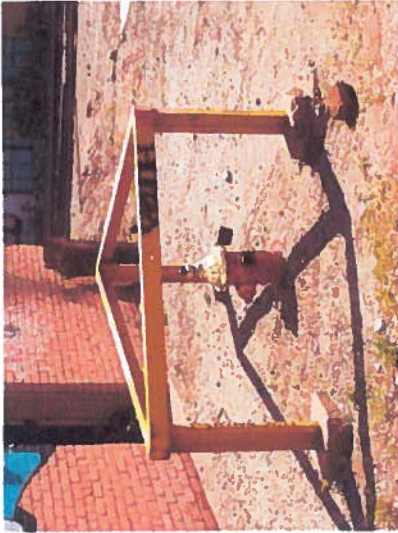
FIGURE 11: An existing fire hydrant, status unknown, located at the southwest corner of the brick outbuilding is partially buried, an apparent lack of adequate grade control.
