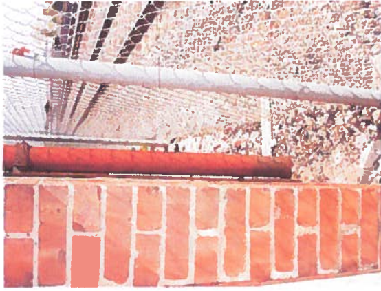
FIGURE 28: Another view of a roof drain on the east face of the Blacksmith Shop as seen through an existing window in the building. It is unknown if this pipe connects to an underground system or a simple dry well. Regardless, this is an existing condition that has likely been serving the site for many decades.
