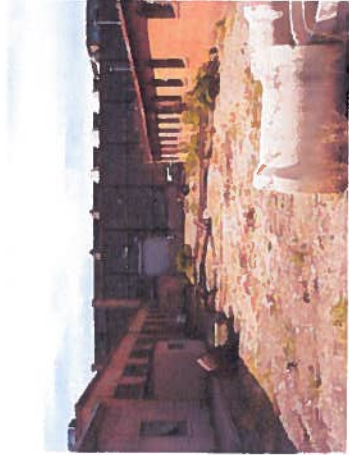
FIGURE 6: The area between the buildings also exhibits poorly defined drainage; the Boiler Shop appears in the background.
