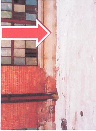
FIGURE 16: Existing roof drain near the northwest corner of the Blacksmith Shop appears to discharge below grade. This location is a de facto sump; the high water mark is observed on the face of the building. The white chalky residue is believed to be washout from the manufacture of movie props.
