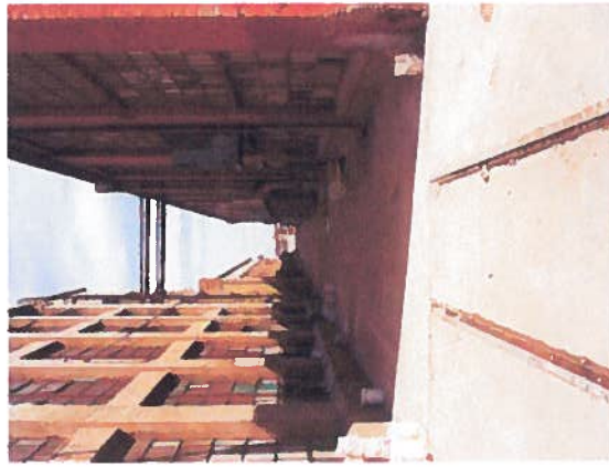
FIGURE 15: The narrow alley as viewed from the south continues to depict a condition absent of positive drainage. An outdoor urinal is located at the midpoint of the east (right) side of this space. It is unknown where this abandoned facility drained or drains.
